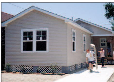
Habitat for Humanity constructed its first all-treated wood home in New Orleans. The raised floor design (1050 sq. ft.) called for 8,500 board feet of KDAT Southern Pine lumber and plywood.
