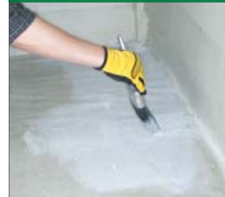
Apply a sealer to the concrete to minimize moisture transfer. Spread it evenly and work it into the surface with a stiff-bristled brush.
