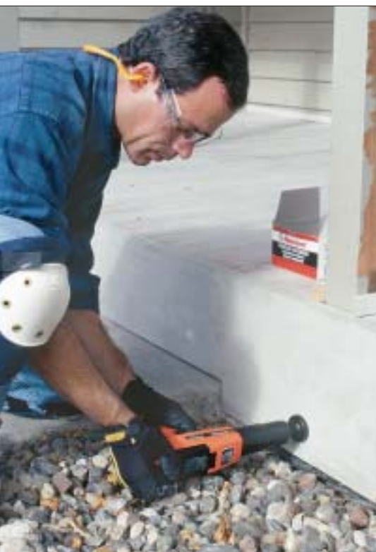
Because the skirt board is decorative, not load-bearing, we used a powder-actuated nail gun to fasten it to the concrete. Although it is flush against the concrete, there is enough space between the board and concrete to allow drainage.
