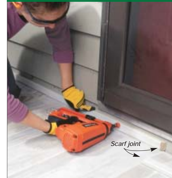
For the trim, we used 1x2 pressure-treated wood painted with porch enamel. A cordless finish nailer made installation easy, and a scarf joint disguised the seam between two long pieces of trim.
